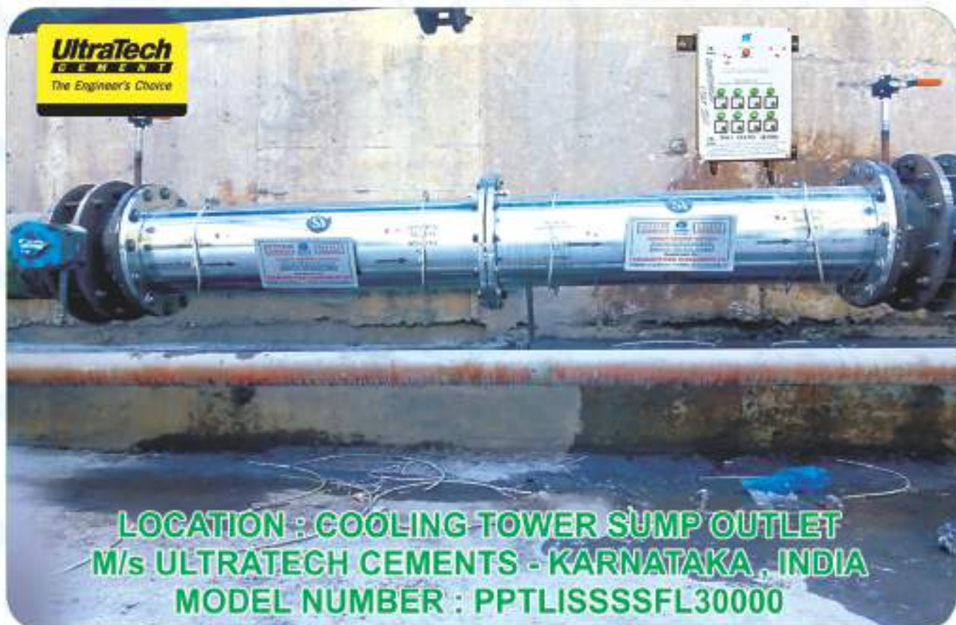
LOCATION : COOLING TOWER SUMP OUTLET M/s ULTRATECH CEMENTS - ANDHRA PRADESH , INDIA MODEL NUMBER : PPTLISSSSFL30000
