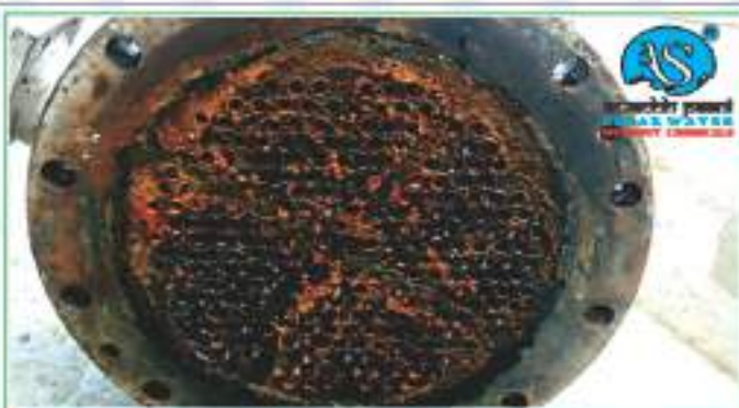
Before installation At Heat Exchanger
