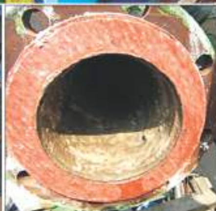
After I.S.S Installation
