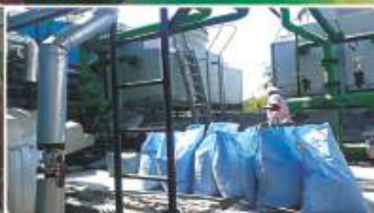
Using the “Instant Solvent Softener” they get good results in few months. The man is cleaning the Cooling Tower area after descaling
