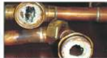
The pipes are blocked due to scaling then the time of water flow increased
